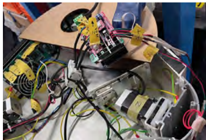
Fig. 2. Wiring of the RAMPS 1.4 shield with printer motors.
